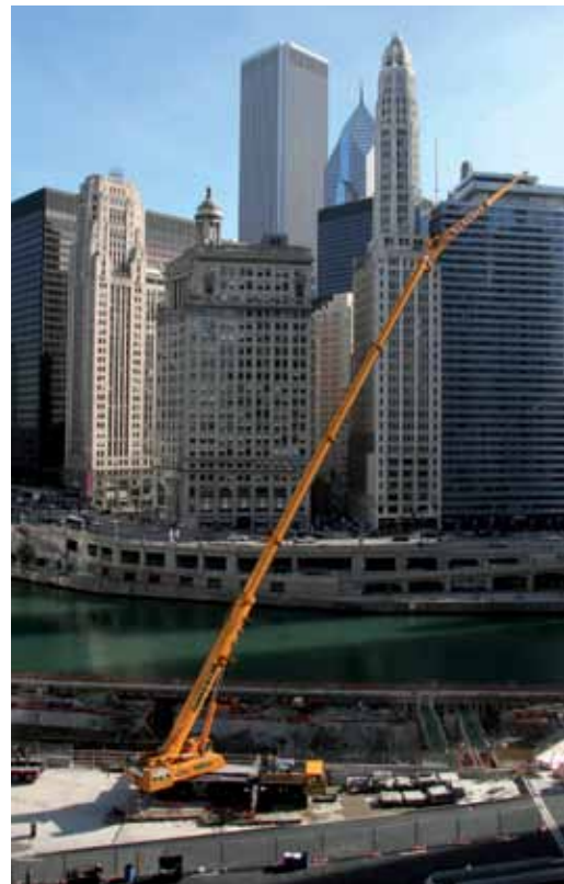
Imperial Crane Services worked on the Trump Tower project in Chicago. The company used its 300-ton hydraulic truck crane, a Liebherr LTM 1250, to erect a massive tower crane exceeding 1,000 feet in height. Crews worked in very tight traffic conditions along the Chicago River in the heart of downtown Chicago
